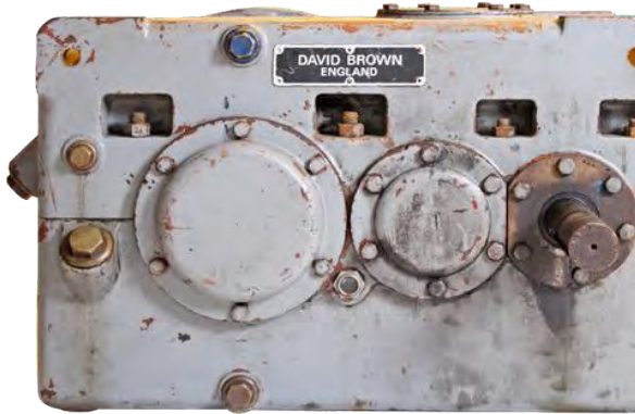
David Brown gear box before refurbishment
