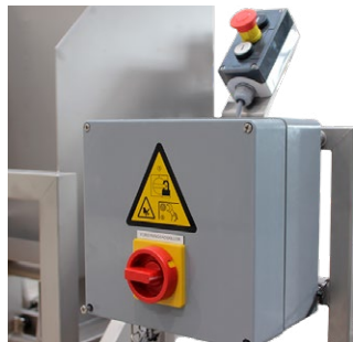
Operator/control panel with emergency stop.
