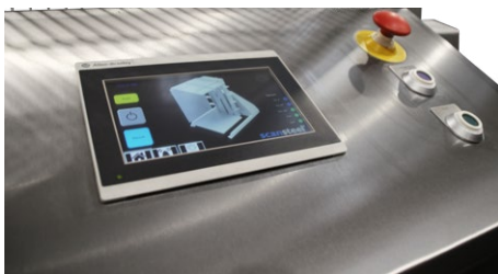
Electrical panel, including touch panel and manual buttons. The cabinet is certified stainless steel, AISI 304 execution.
