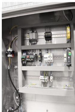
View inside electrical panel.
